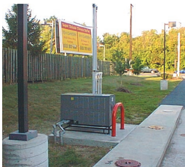
Figure 4: OPW's membrane unit.
