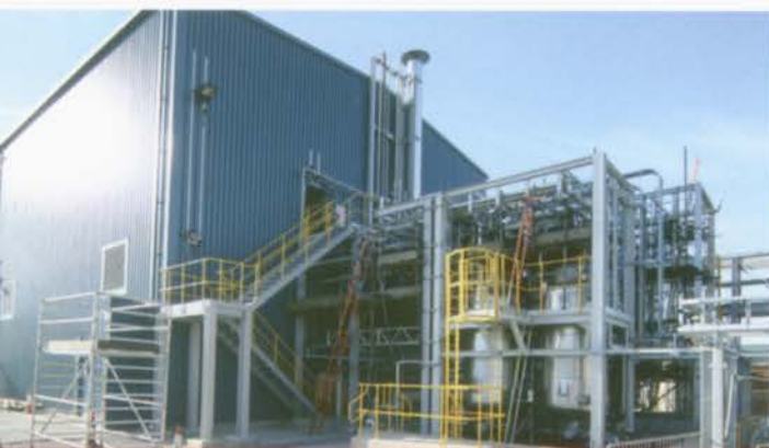
Butamax's 40,000 gallon-per-year technology demonstration plant in Hull, UK.
